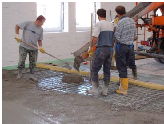
Fig. 3 Repair layer. The mesh could be placed parallel to pouring of the concrete
